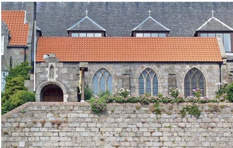
Right: the Founder's Aisle, St Margaret in the Gallowgate, viewed from the south.
