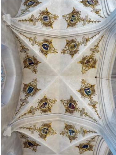
Above: ribbed vaulting to the north aisle, the decorative plaster castings at each bay representing eight American states of the Union.
